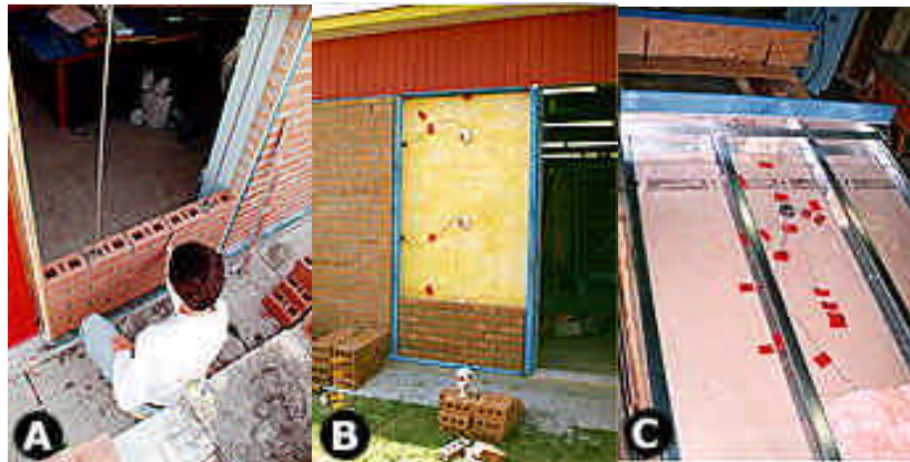
Masonry Construction (A), Wall Instrumentation in Place (B) and Wall Assembly (C)
