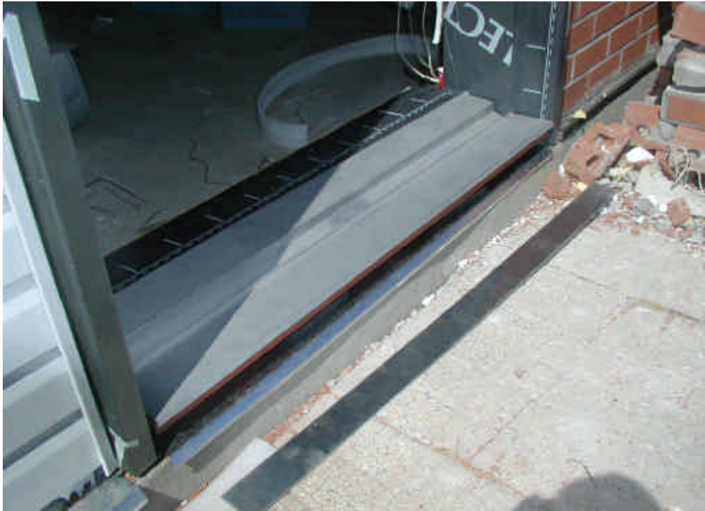
The Base Detail Can be designed to Collect Drainage Normally Directed to the Exterior
