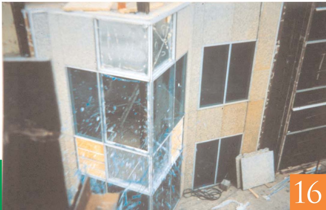
Fig. 19 – Glass Failure during Curtain Wall Testing
