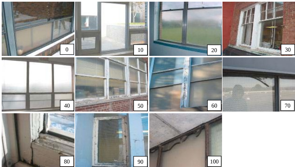
FIGURE 3 Ranked pictures at different deterioration levels
