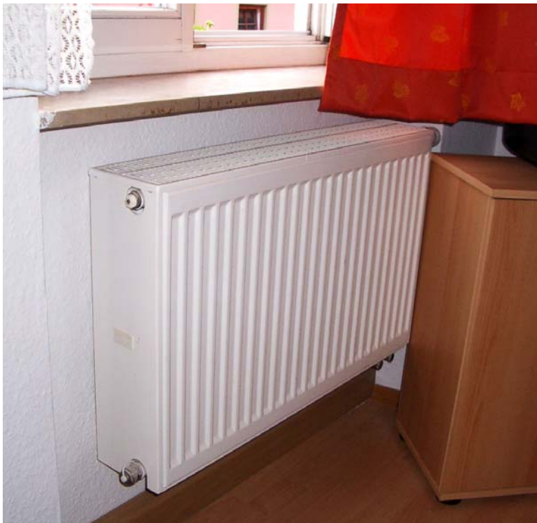
A hot water “radiator” terminal unit that actually transfers most of its heat to the room by convection
