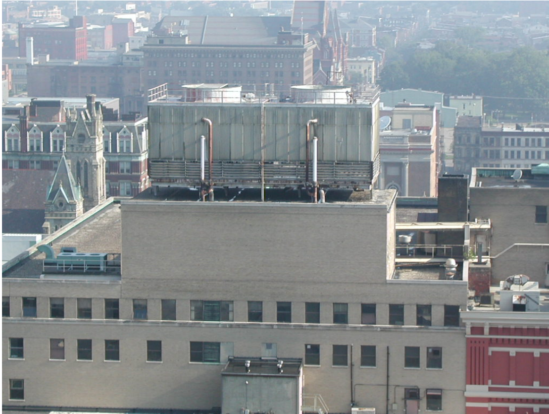
A cooling Tower for a Large Cooling Load
