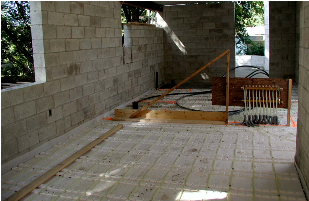
Radiant floor heating tubes over insulation
