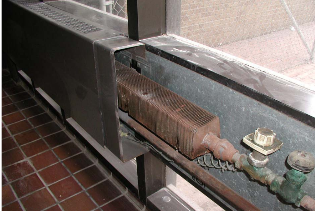
A commercial finned convector cabinet with cover removed and supply pipes visible
