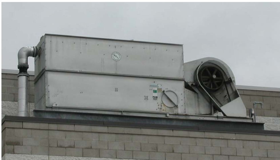
A more common shape of a cooling tower
