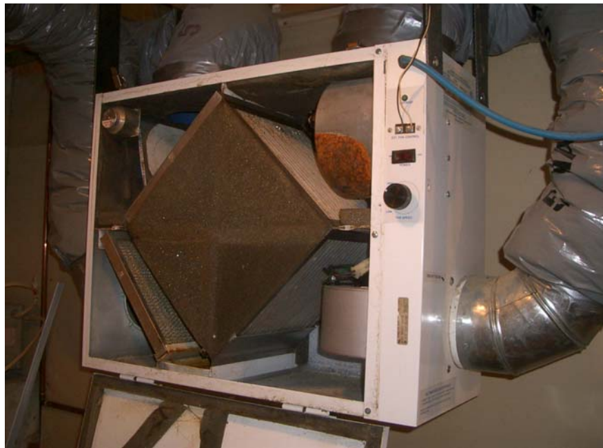
A 15 year old HRV with cover open – note diamond shaped heat exchange core, dual fans (on right side) and insulated ducts for supply and exhaust to exterior
