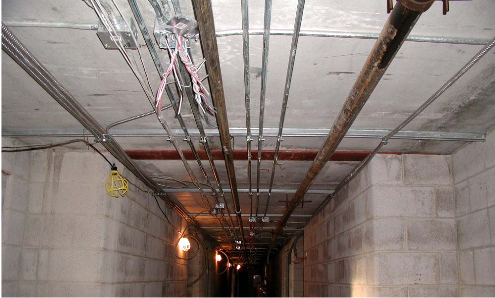
Service (power, communications fire suppression water) distribution in corridor of an apartment building
