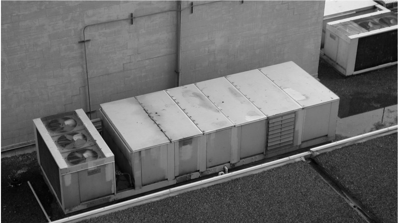
Rooftop packaged units contain heating, cooling, filtration, and fresh air ventilation in one unit.
