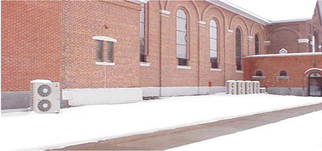
Outdoor Condenser Units
